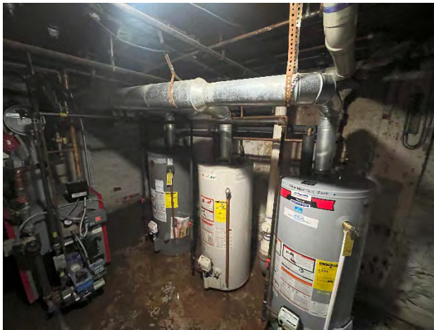
Hot water tanks (one installed 11/12/2024)
