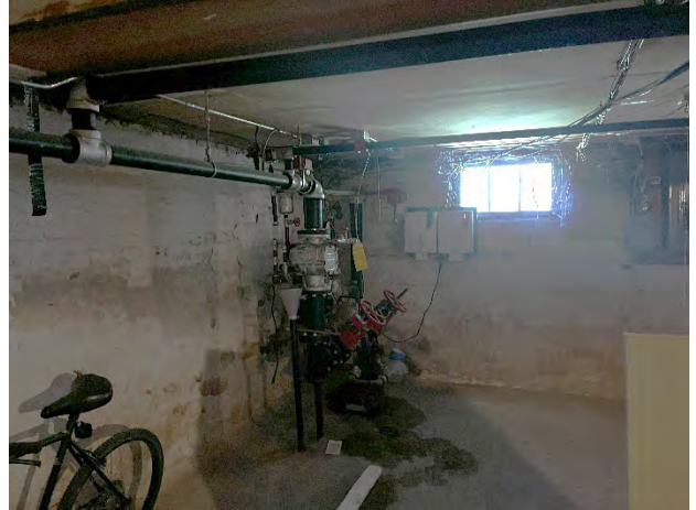
Wet sprinkler system
