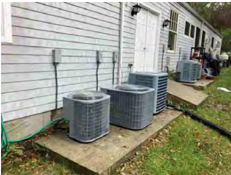
Central a/c compressors
