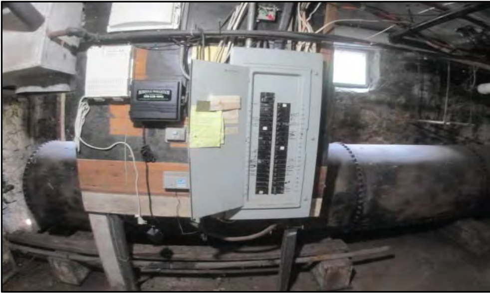
49 Elm St ELECTRICAL BOX basement
