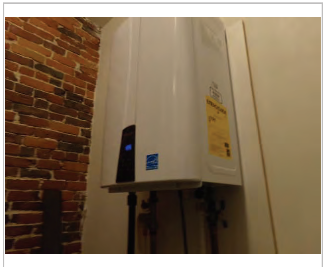
INTERIOR - HOT WATER HEATER
